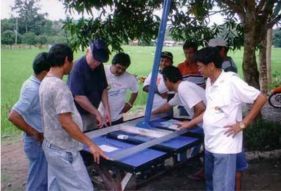
Eric Jensen assembling a solar pump in the Philippines for a school
