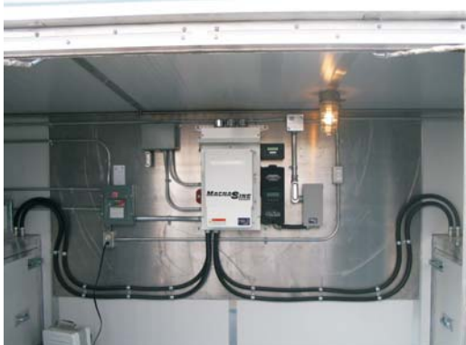
INVERTER + POWER-BOARD ASSEMBLY
